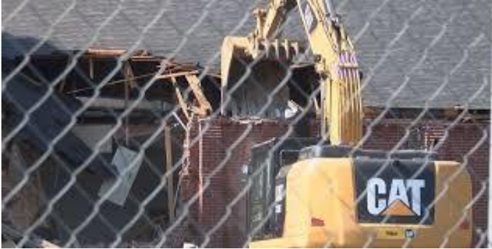
Blessed Sacrament Parish Hall Demolition North side of Building, facing the church. View is looking south from the church. Picture Source: KAIT-TV, June 9, 2016
