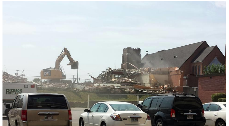
Blessed Sacrament School Demolition Back of Building. View is looking west from St. Bernard's Picture Source: Unknown
