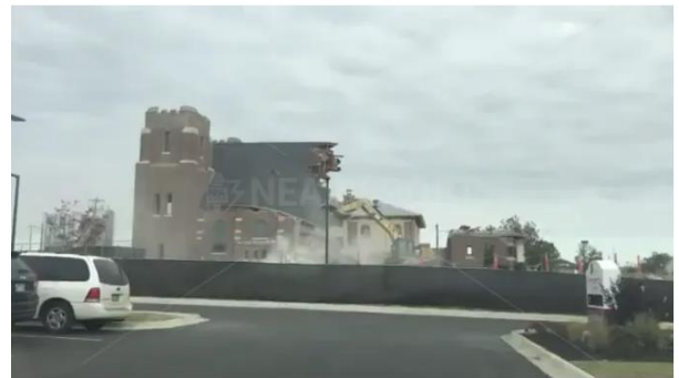
Blessed Sacrament Church Demolition South side of Building. View is looking north from the former parish hall site. Picture Source: NEA Report, October 31, 2017
